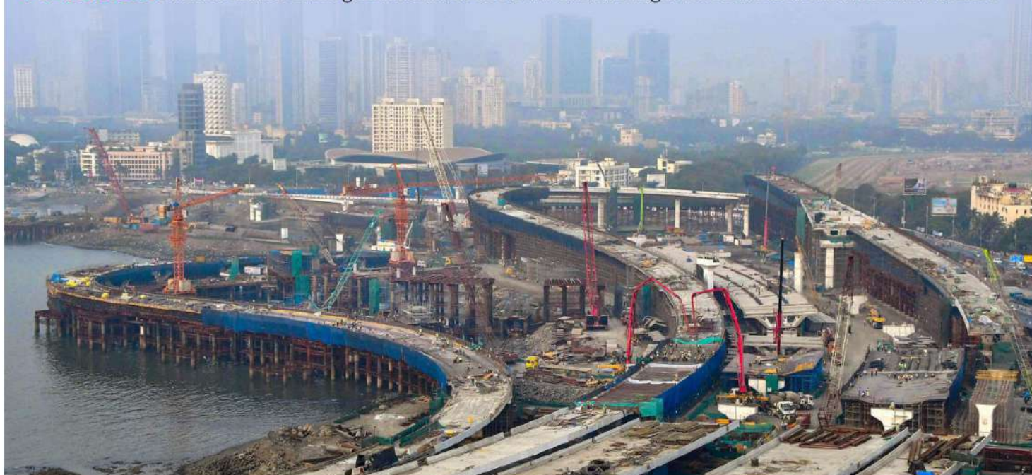
BIG BOOST. The construction of Coastal Road Project is underway in Mumbai. The government has proposed a 25 per cent higher allocation at ₹2.70-lakh cr for roads compared to FY23 RE
